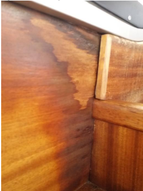
Fig 4 - Signs of previous water ingress
